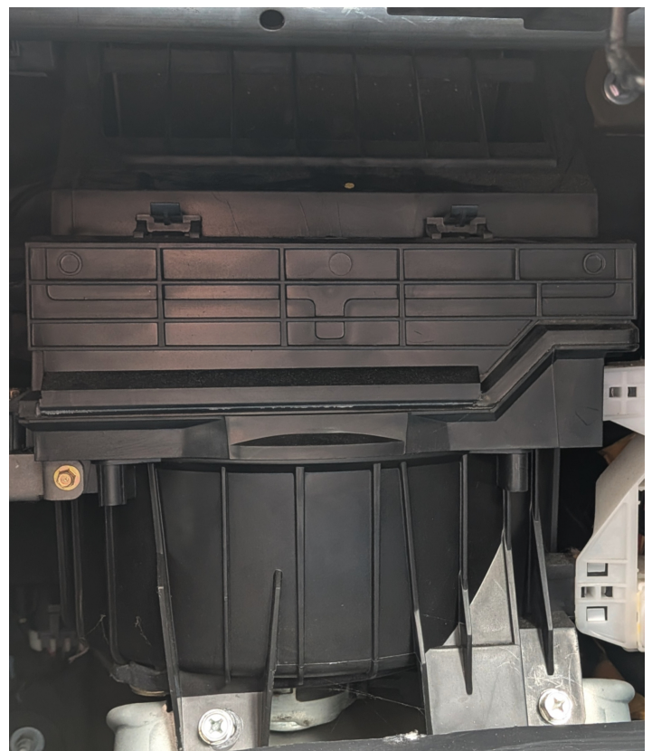
Filter lid closed (Done; Flowing plenty cold air!)
